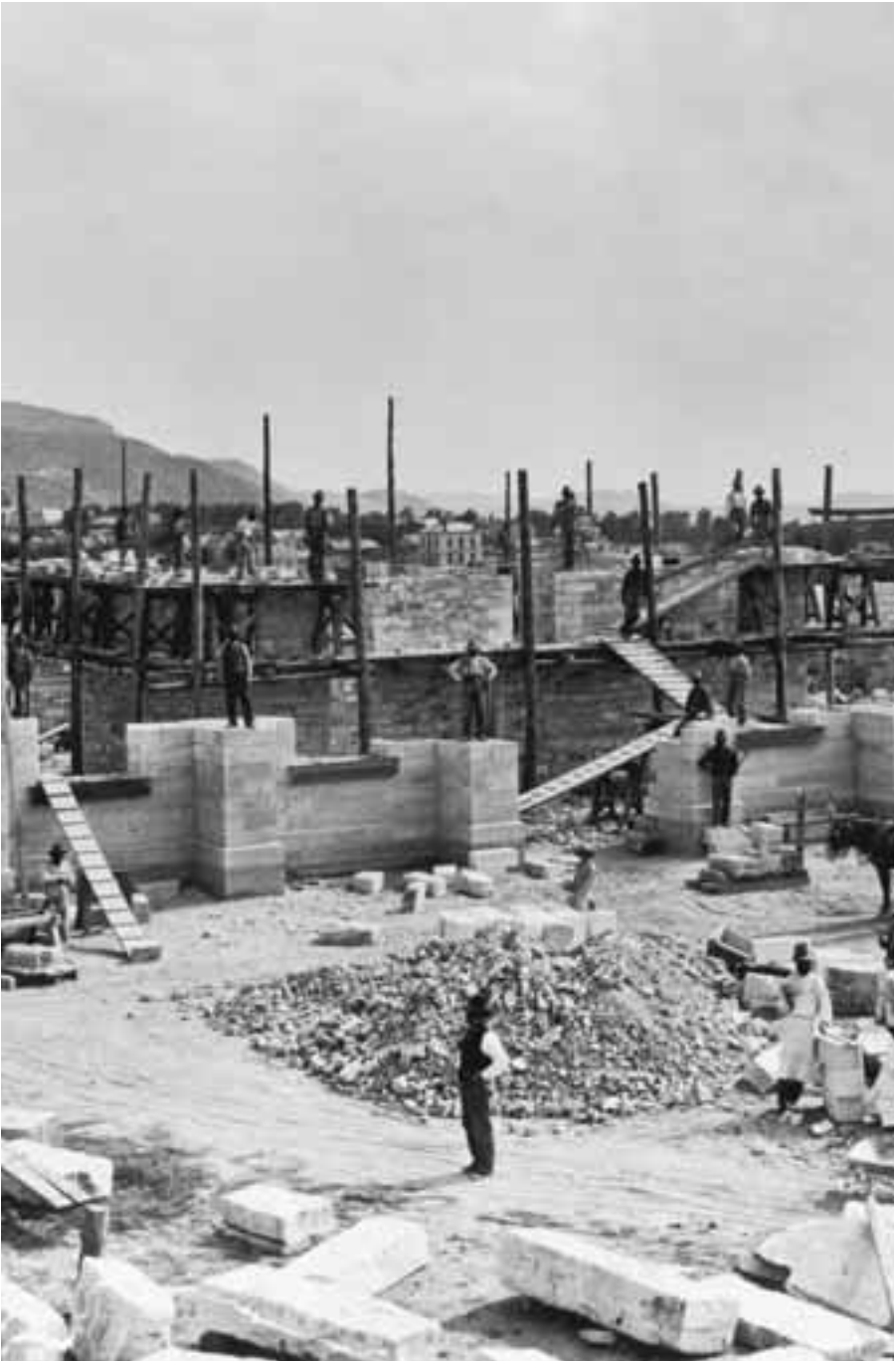
President Brigham Young was known as a great colonizer. He dedicated the site for the Manti Temple (shown here under construction) in 1877.
