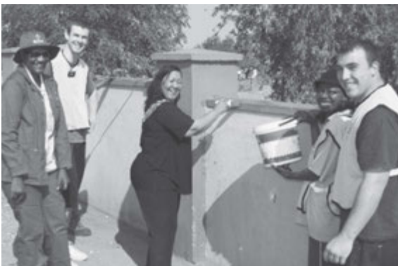
Windhoek Mayor Elaine Trepper paints a portion of the Katutura Cemetery wall while missionaries and others look on.
